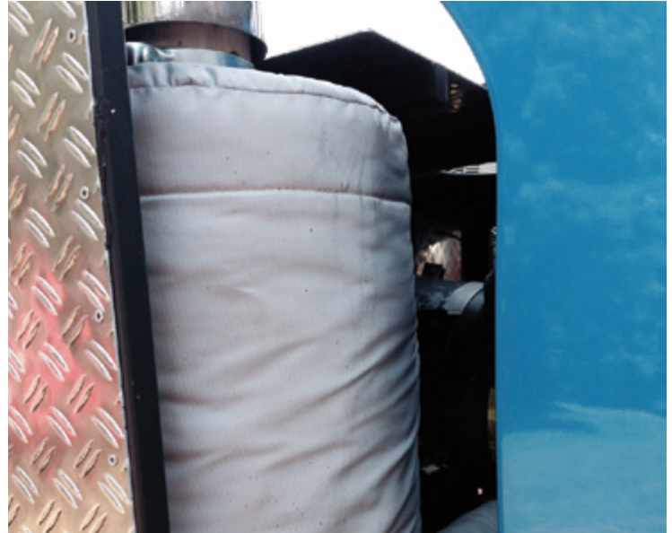
Insulation of a particulate filter
