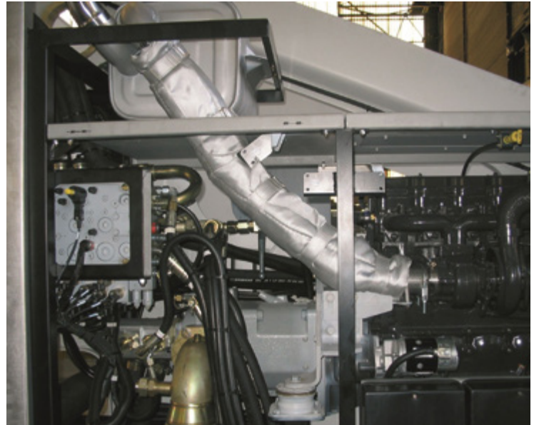
Exhaust gas insulation
